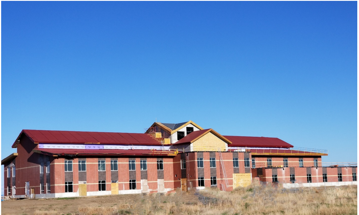
The two-story new school is nearly complete on the outside. On the inside, sheet rock, elevators, stairs, and rooms are looking more and more like a magnificent school.
