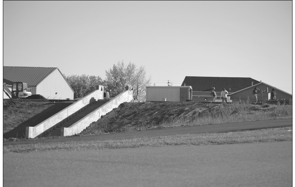
Here is a side view of the Veterans Memorial Wall. Workers are diligently working hard while the weather is good.
