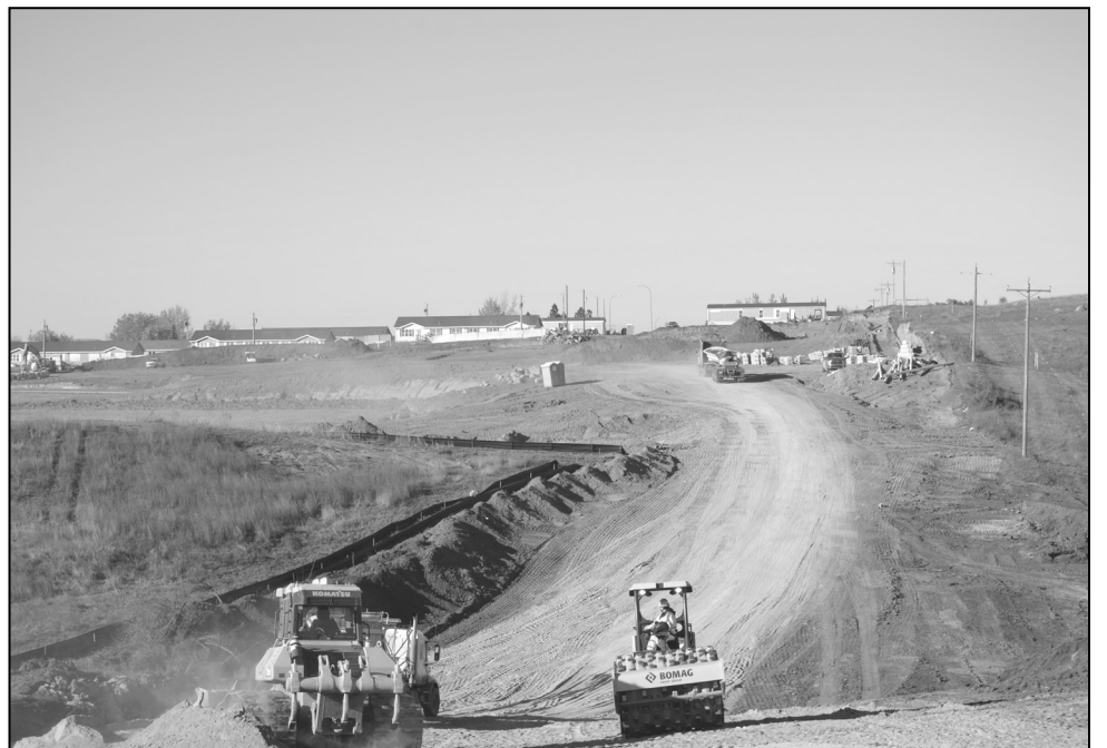
Construction is being done on a daily basis getting as much done as they possibly can.
