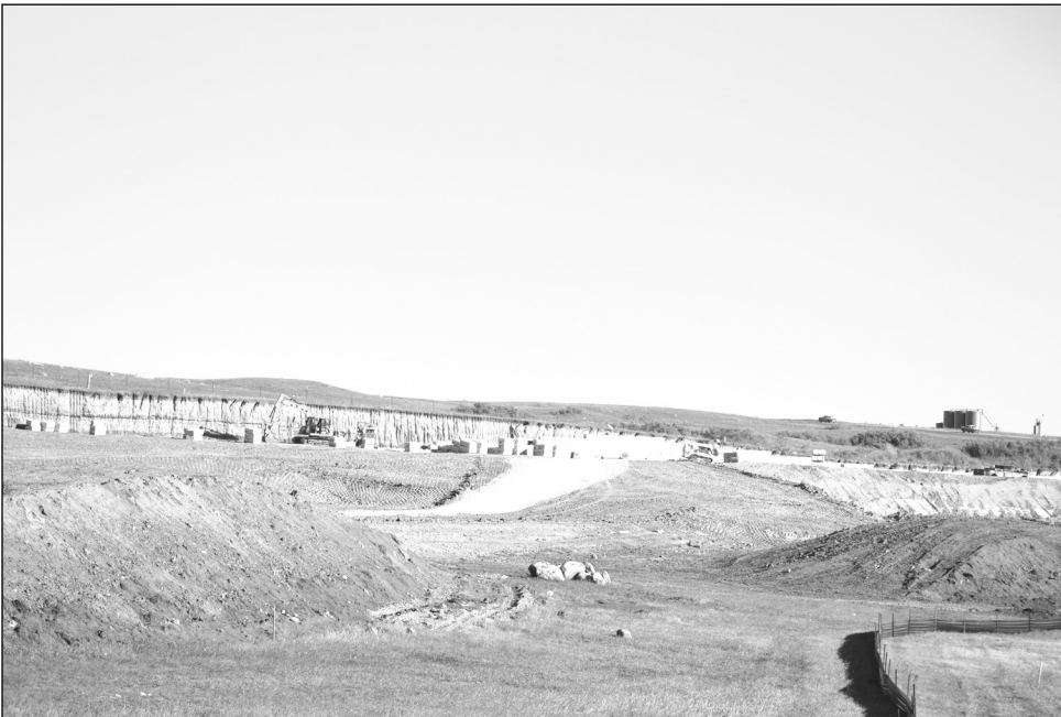
Here is another angle they have cement blocks piled up for building.
