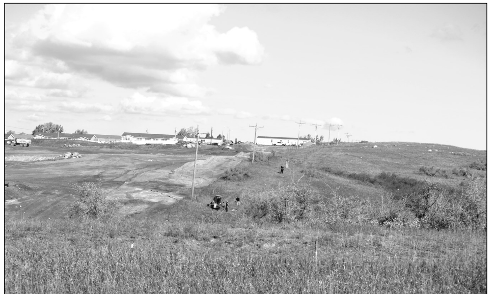
Steel pipe needs to be driven into the ground the workers on the side are walking along the lines of where the steel pipes goes.
