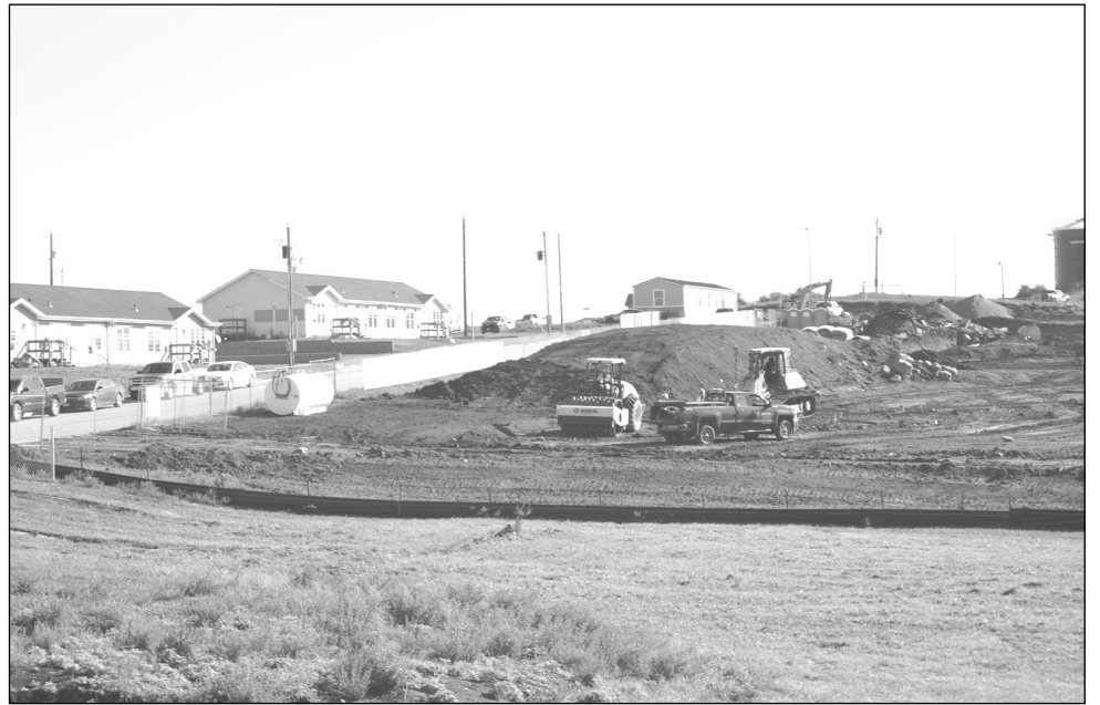
The ground work begins from here and extends out to the road on route 12. Our community is slowly making changes.
