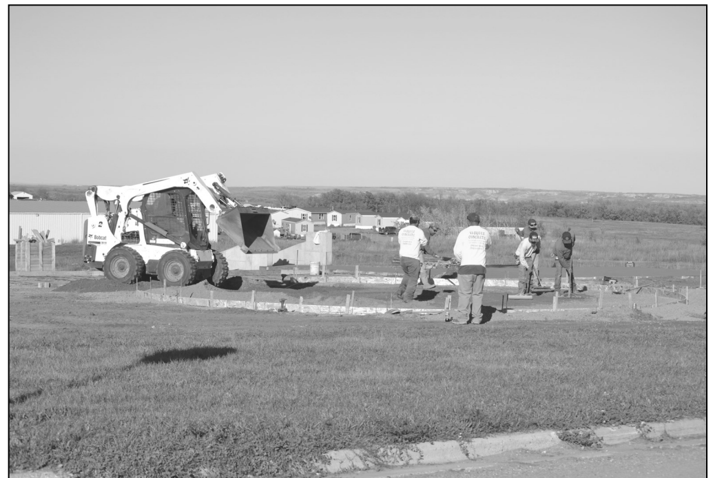
Workers were busy breaking ground and have a layout of the Veterans Memorial Wall.
