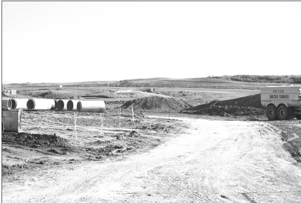
Concrete footing and foundation work will start at the south half of the community center.
