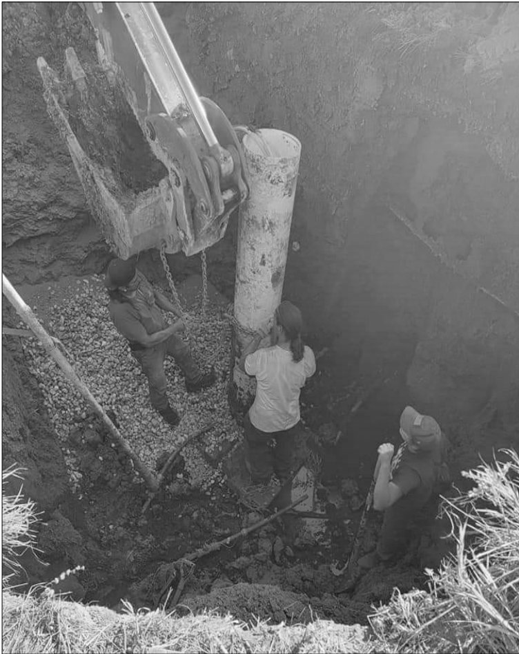
Here you can see the workers putting the chain around the pipe so it can be lifted.
