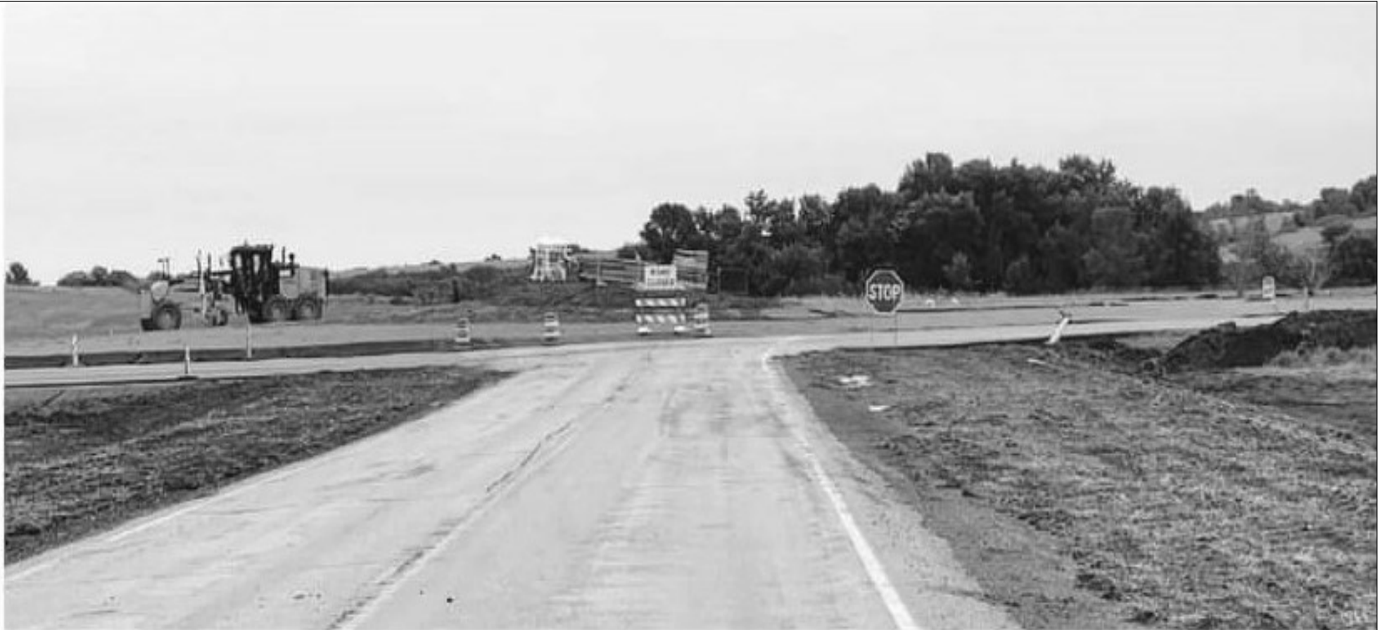
Construction of roundabout near Mandaree, at the junction of highway 22 and highway 73.
