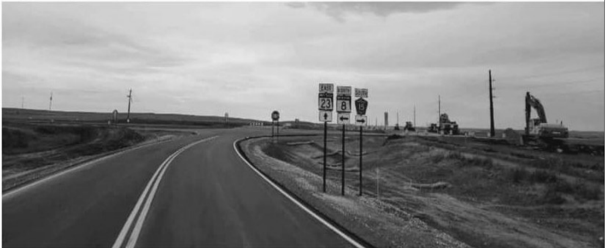
Construction of roundabout near New Town at the junction of highway 23 and highway 8.
